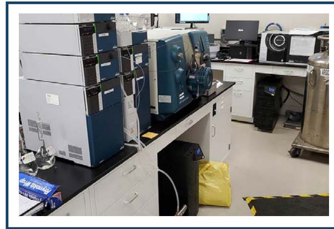
Battery Backup Power, Inc. 6KVAs Protecting Lab Instruments
