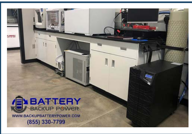
Battery Backup Power, Inc. BBP-ADV-10000 10KVA UPS Protecting Agilent 7900 ICP-MS
