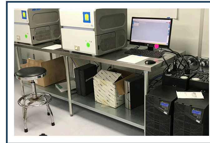
Battery Backup Power 6KVA Protecting PCR Instruments At COVID Testing Lab
