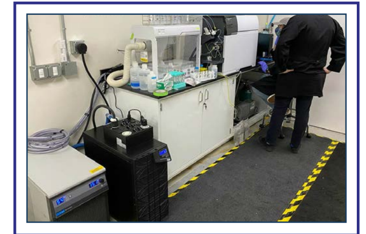
Battery Backup Power 10KVA Protecting Agilent ICP-MS
